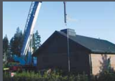
Pump Service Crains
